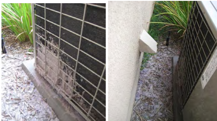
Figure 11-35: Noncompliant Condensing Unit Clearance from Dryer Vents
