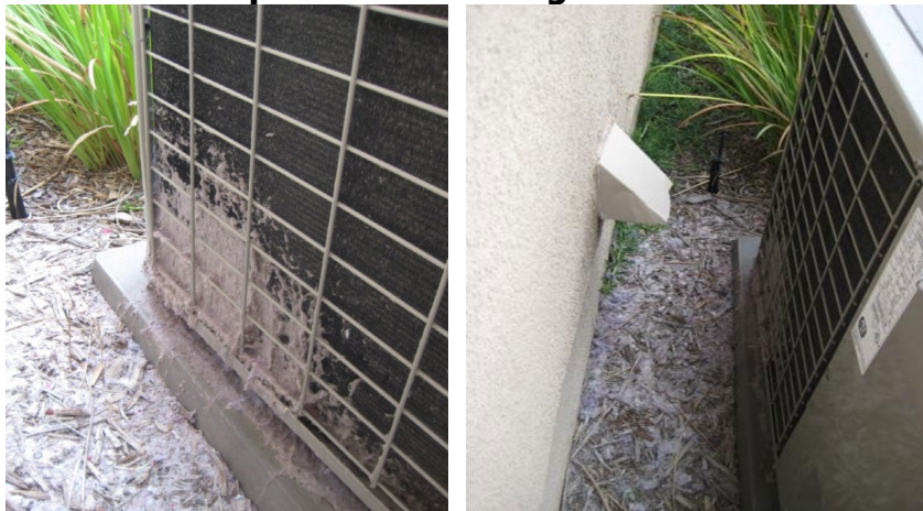
Figure 4-2: Noncompliant Condensing Unit Clearance from Dryer Vents
