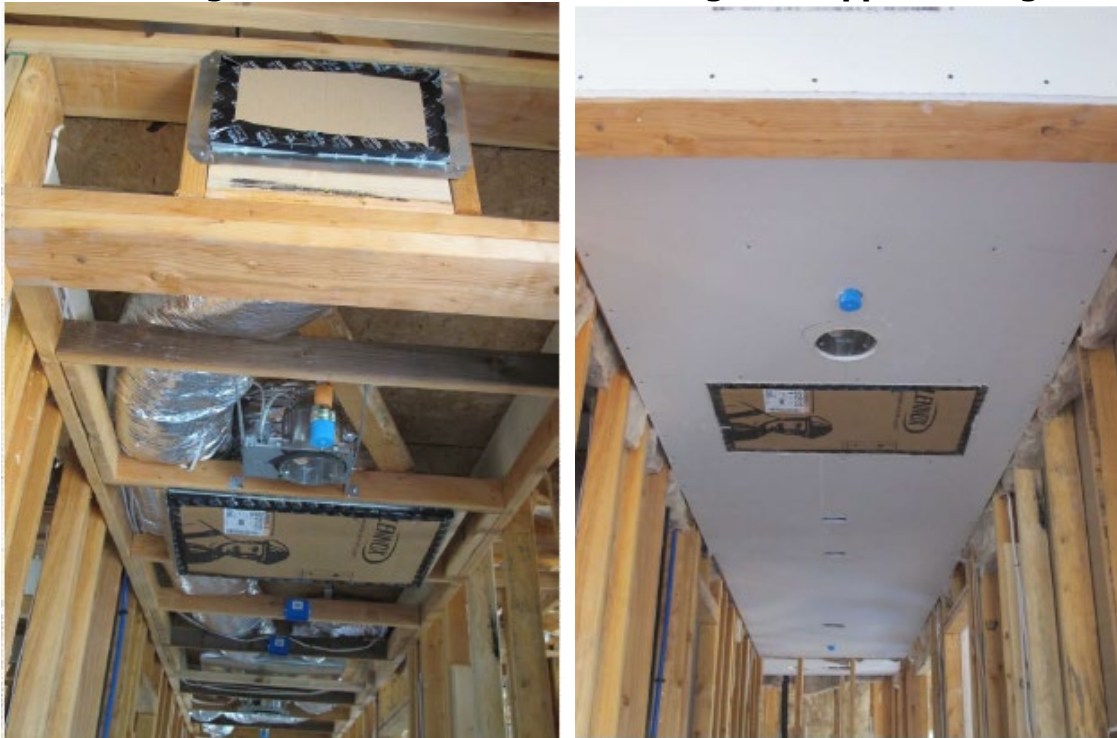
Figure 4-11: Ducts Routed Through a Dropped Ceiling
