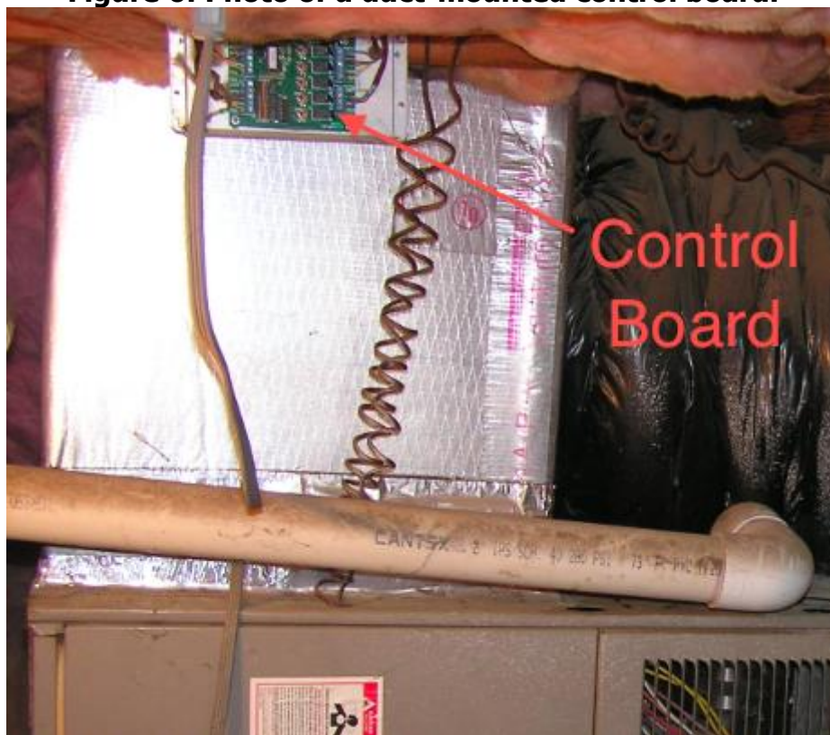
Figure 6: Photo of a duct-mounted control board.
